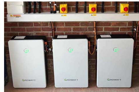
Home Battery Storage
